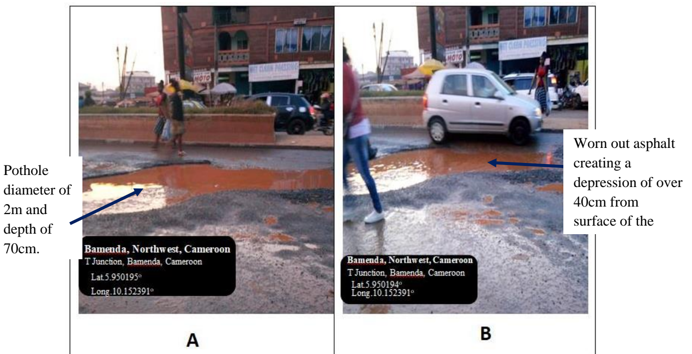
Figure 7: The poor surface state of most streets characterized by potholes
